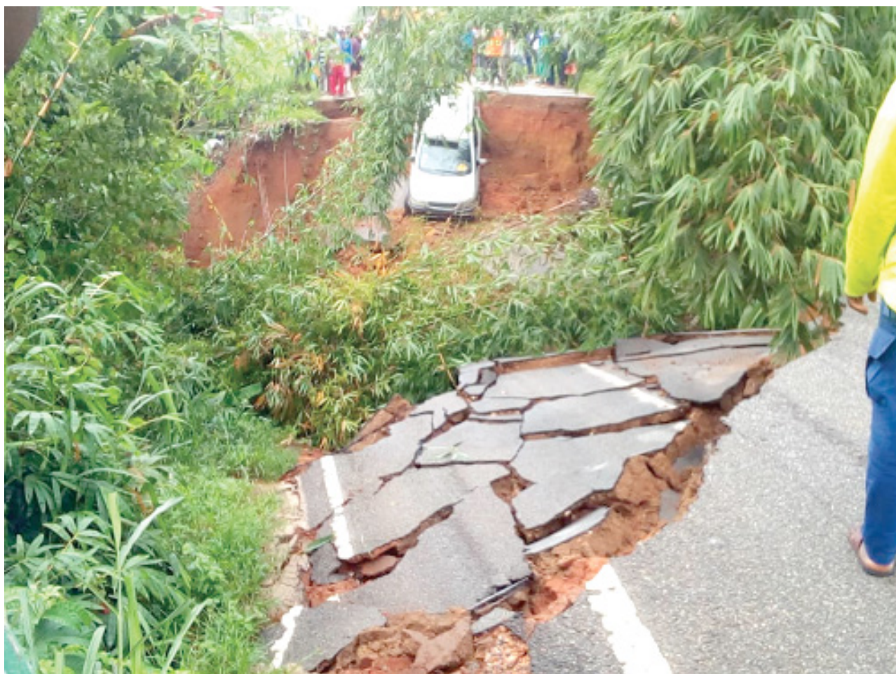
Plate 8. The road linking two communities in the Ellembelle District to the Apimanim-Elubo highway washed away after heavy rains and flooding in 2021.
